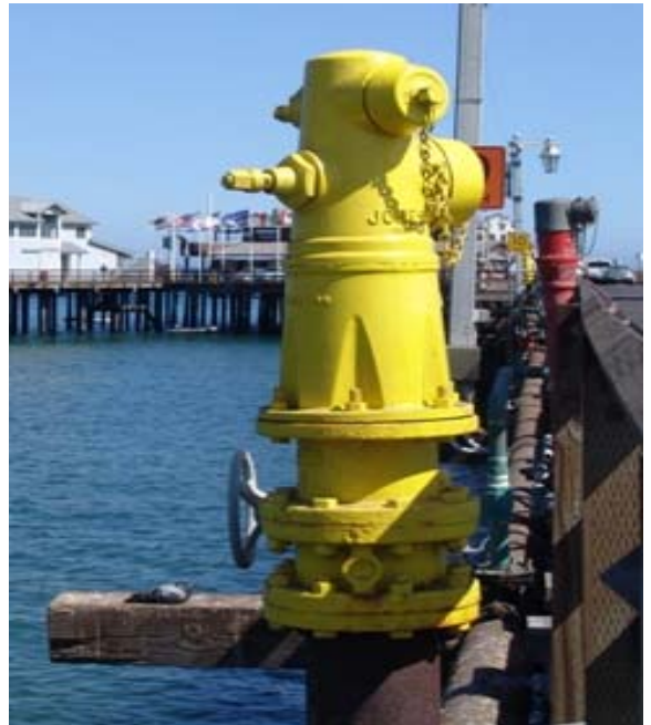
Hydrant in Santa Barbara
